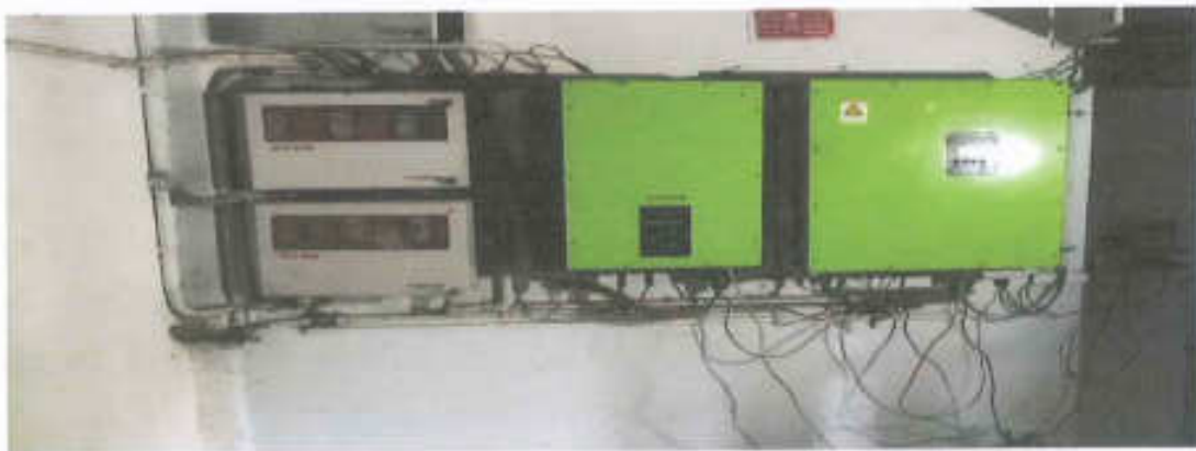
Pictures of Solar Power Plant
